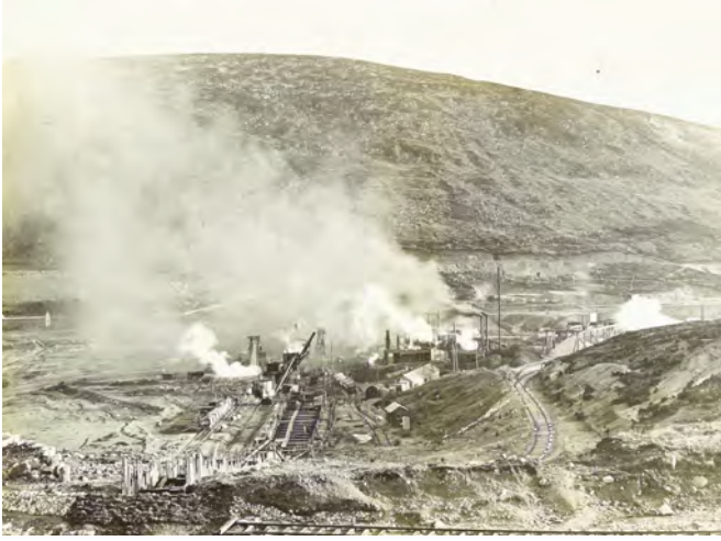
The landscape on fire; work underway on the massive and ambitious project
